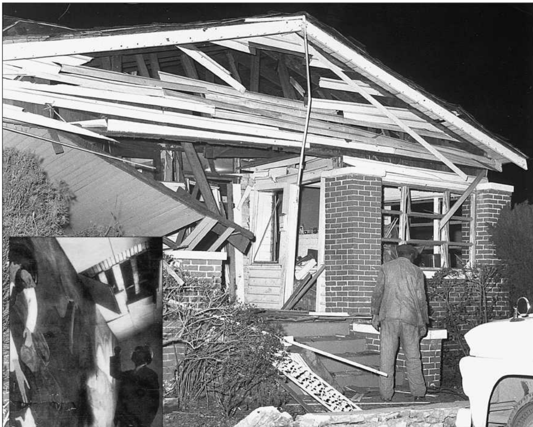
"Bomb damage at Bethel Baptist Church is viewed by Rev. V. C. Provitt, Blast occurred last December," Saturday Evening Post, March 2, 1963, page 15.
